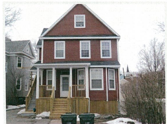
Figure 2 – Under the Rental Rehabilitation Assistance Program, we partnered with a landlord to upgrade 3 affordable rental units. New siding and windows were installed and exterior porches and stairs were replaced.
